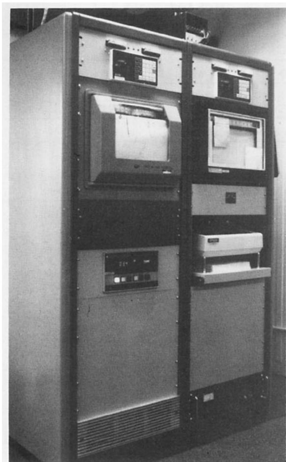
FIG. 4. Two CAMS shown at the top of the equipment racks in a typical installation. The printer that is shared by the three CAMS is located in the middle of the right-hand rack. The RS-232 switch used to select the individual CAMS is located immediately above the printer.
